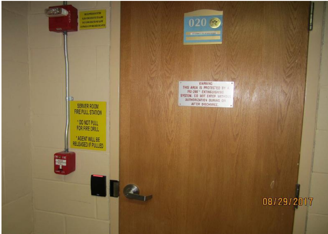
Figure 13: Entrance to the secured computer server room requires a badge for access.
